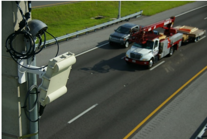
Figure 8: Microwave vehicle detection system
